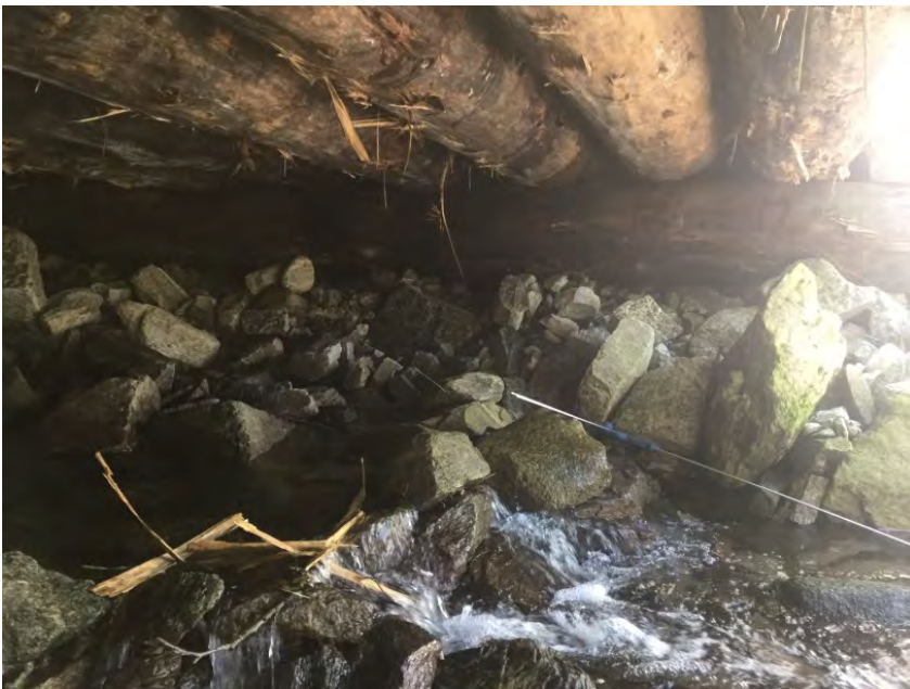
Eroded riprap downstream left bank
